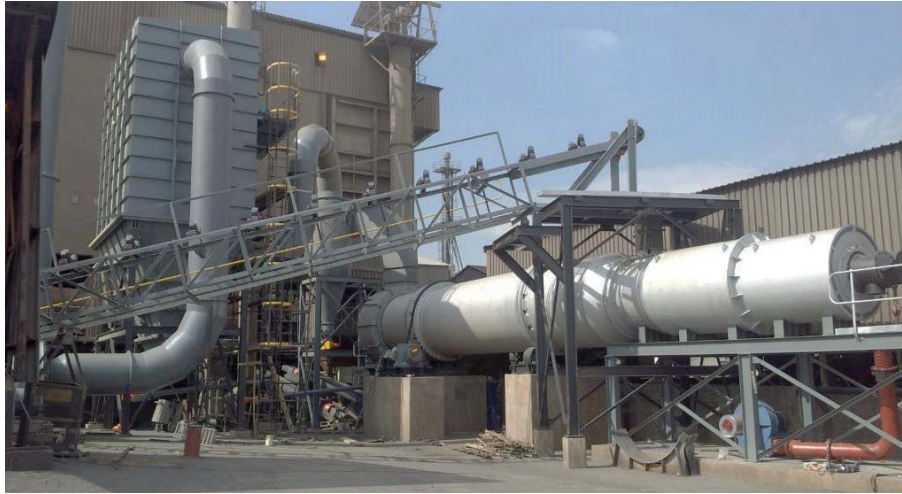
Figure 2: A Rotary drier and its off-gas cleaning system
